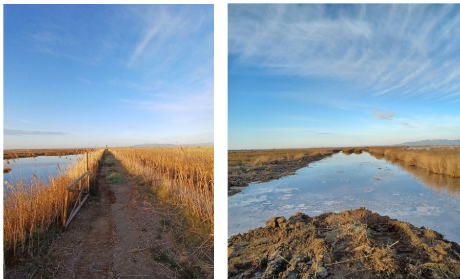
Figure 20: Alfacada Lagoon before (left) and after (right) the removal of the dike. (Source: EURECAT)
