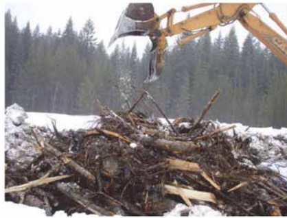
Fig. 6. Excavator building forest residue piles (photo by J. G. Archuleta.) in the USA (Page-Dumroese (2017))
