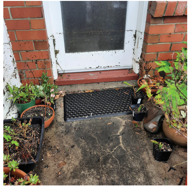
Figure 5. Flood level on Janene's front door, 28 January 2023. Image courtesy of Janene Smith. © All rights reserved.
